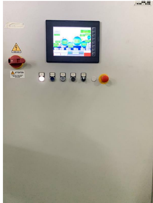
Figure 2 - Horner eXL10 PLC/HMI in place on the machine's cabinet
