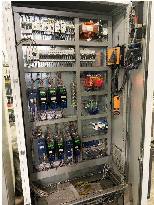
Figure 1 - Inside of the cabinet of the carding machine
