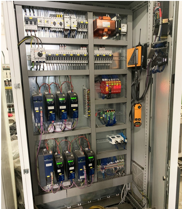
Inside of the carding machine cabinet (Source: Horner)
